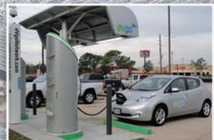
8) EV Filling Station Completion date:
