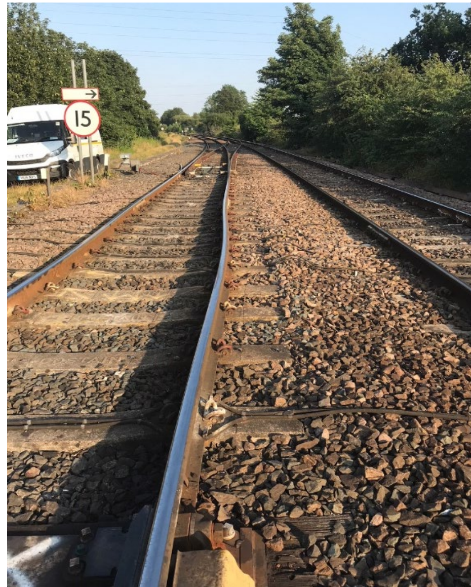
Heat (Buckled Rail) - Oakenshaw Jn – 24072019 - Brett Hill (Network Rail)
